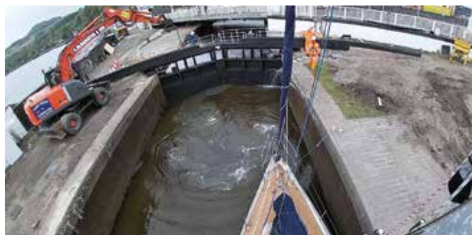
Winter refurbishment had over-run, so an excavator was used to raise the sluice!
